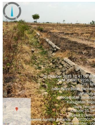
FIGURE 4. Irrigation Channels Heavily Damaged
